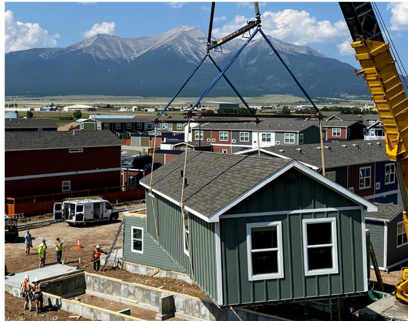
Fading West's factory-produced homes are shipped to their permanent location at costs of up to 25% cheaper than comparable traditionally-built homes, making homes more accessible during a housing crisis. Fading West
